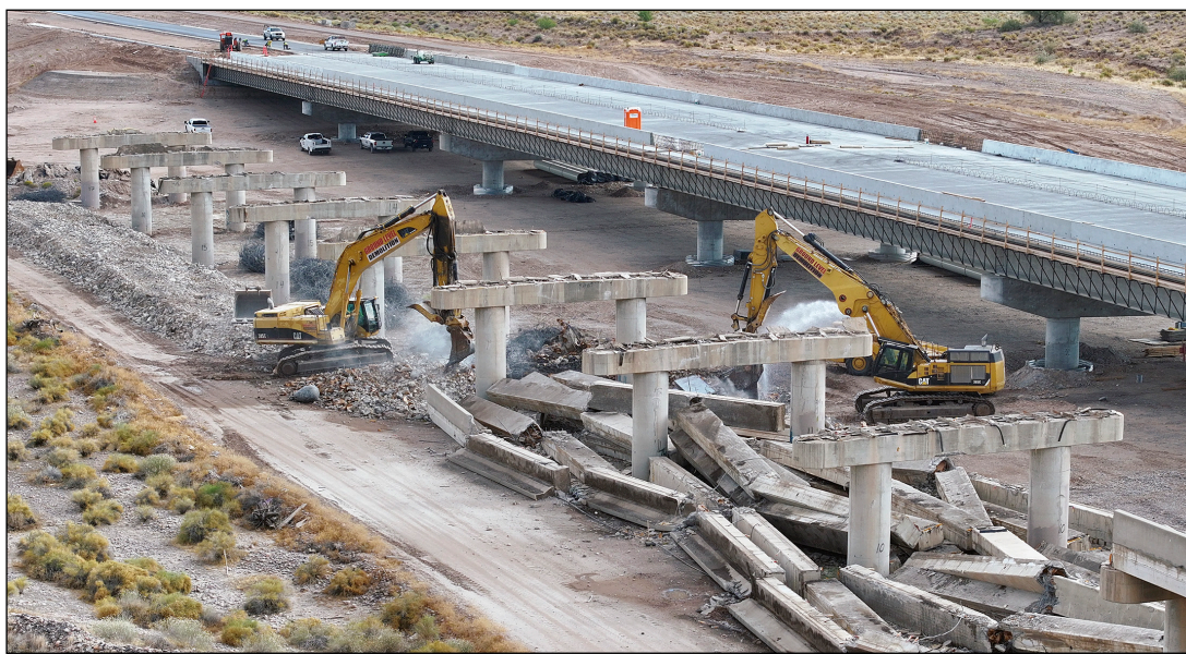
The original Gilbert Road Bridge is being demolished and removed as part of the project construction. Courtesy of Maricopa Department of Transportation
