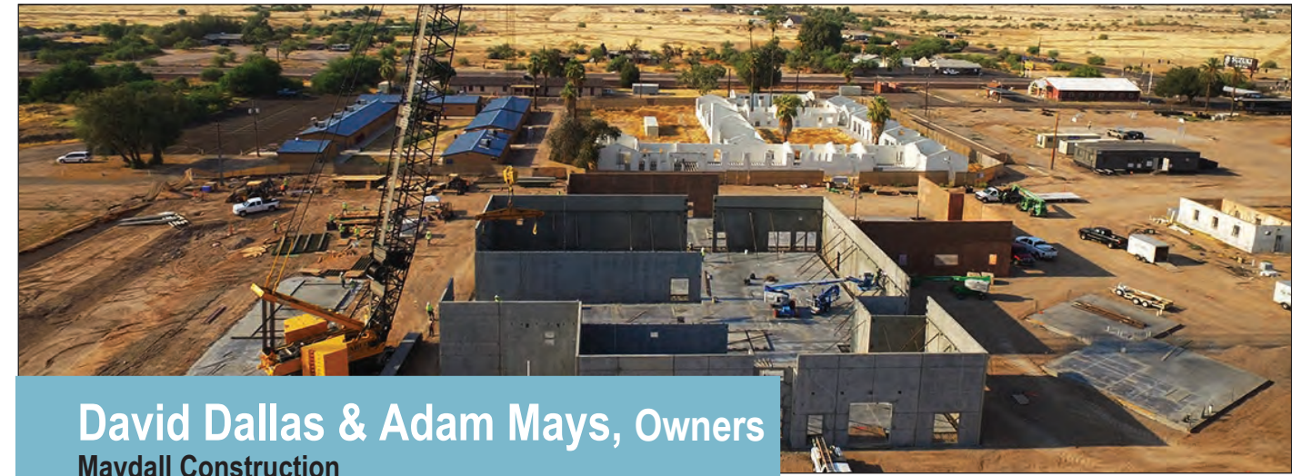
Progress photo of the Cultural Resources Department Repository on Longmore and McDowell. Photo courtesy of David Dallas
