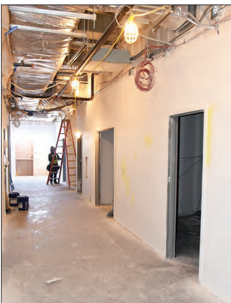
First floor paint, lighting, wiring and flooring are being worked on at the River People Health Center.
