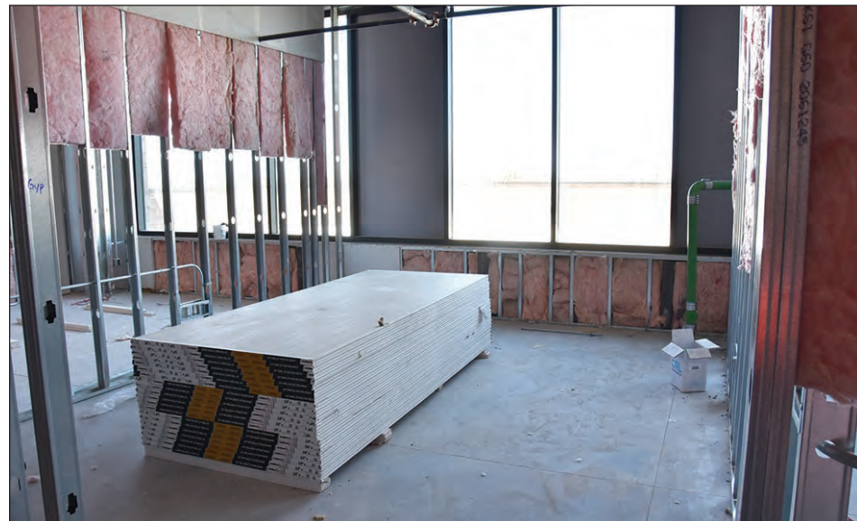
One of the rooms being worked on near the dental portion of River People Health Center on the second floor.
