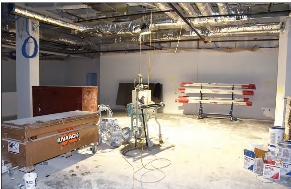
Interior trade construction continues on the first floor of the River People Health Center.
