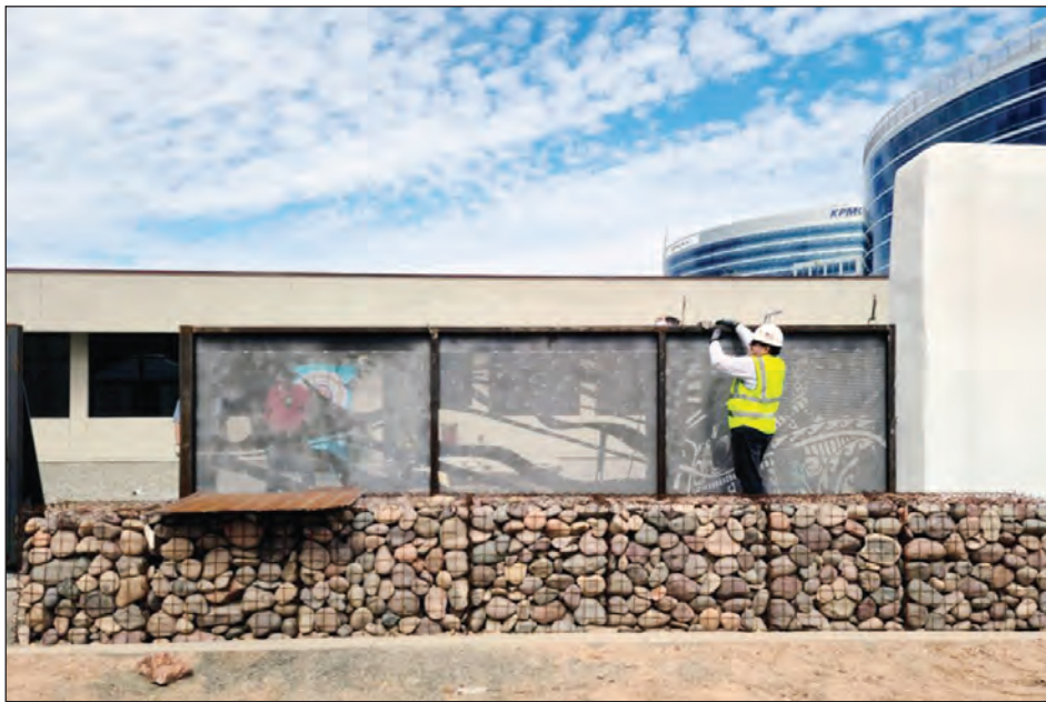
In March, workers install the steel fence that SRPMIC member and artist Jacob Butler designed for the Hayden House. Photo’s courtesy of Jacob Butler
