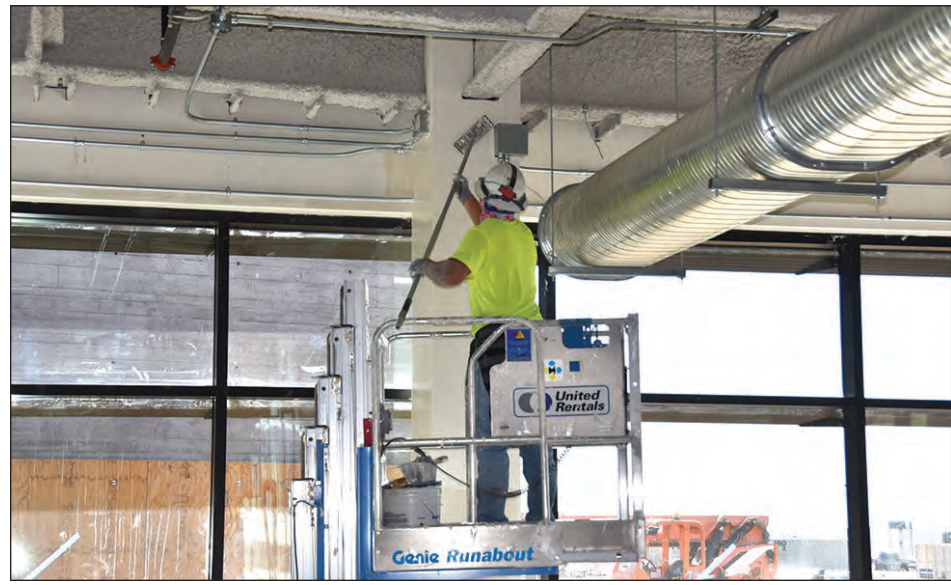
Painting being finished by a crew member on the first floor of the River People Health Center.
