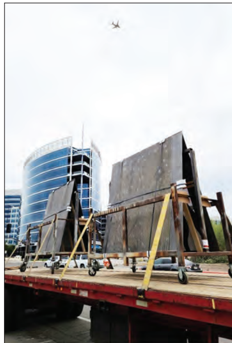
The steel fence panels arrive on a flatbed truck in Tempe to be installed.
