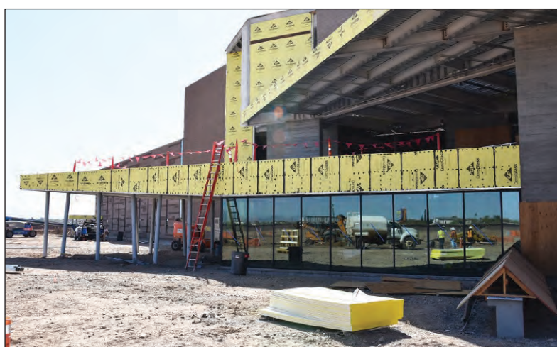
The front entrance to The River People Health Center off of McDowell Road. The next phase for the entrance is work on getting the curb and gutter, asphalt and landscaping shaped up.
