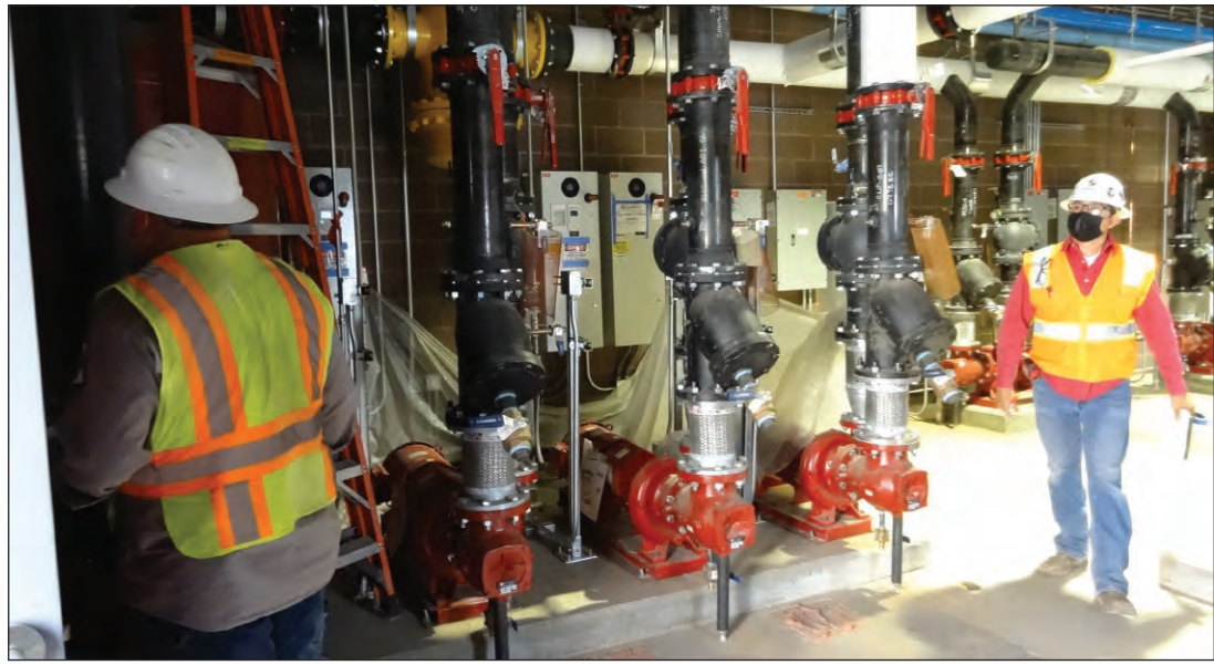
River People Health Center central plant pumps. Photos courtesy of Engineering & Construction Services.
