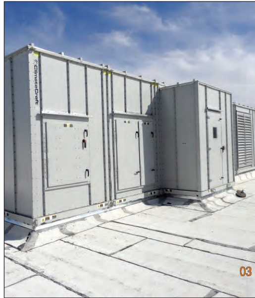
River People Health Center air handler unit. Photo courtesy of Engineering & Construction Services.
