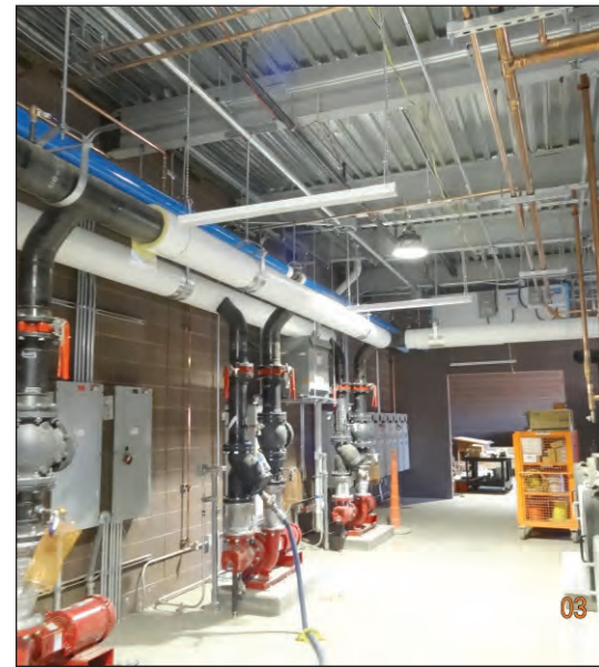
River People Health Center central plant. Photo courtesy of Engineering & Construction Services.
