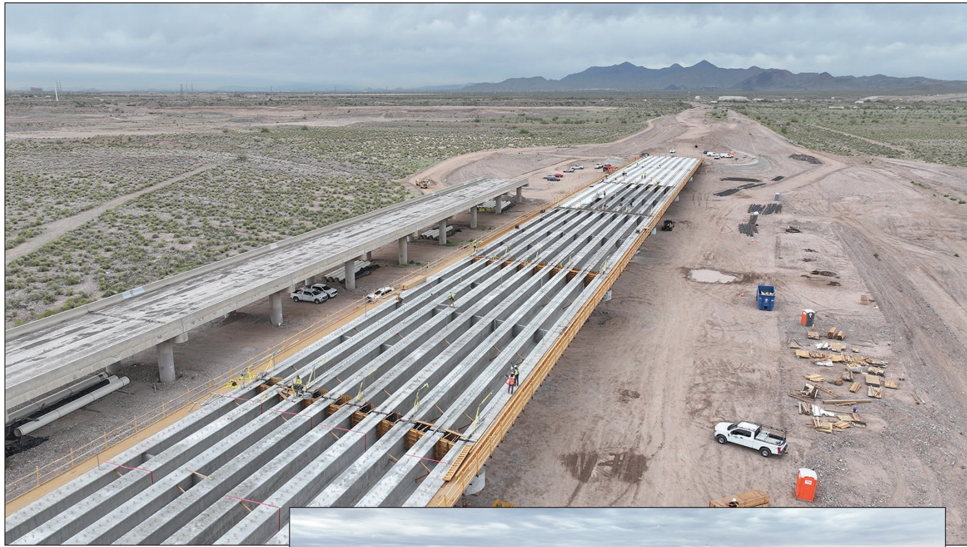
Top: Northbound View of the Gilbert Road Bridge Project toward State Route 87 and SRPMIC.
