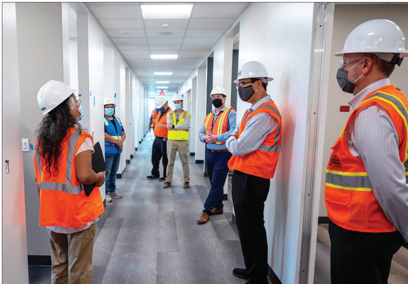
L: Council member Diane Enos has questions for staff during the construction site visit to the River People Health Center in September, 2021.
