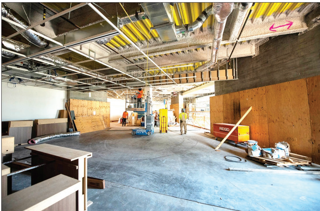
Above ceiling work at 2nd floor lobby of the River People Health Center.
