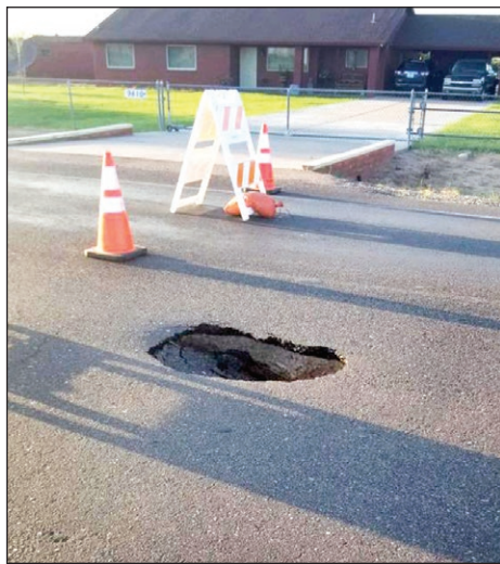
A sink hole appears on Thomas Road after heavy rains. Photo courtesy of Public Works Department
