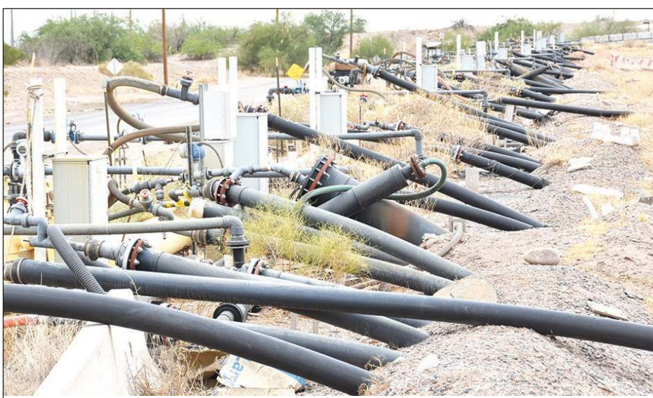
Pipes that collect gas from decomposing waste at the Salt River Landfill.
