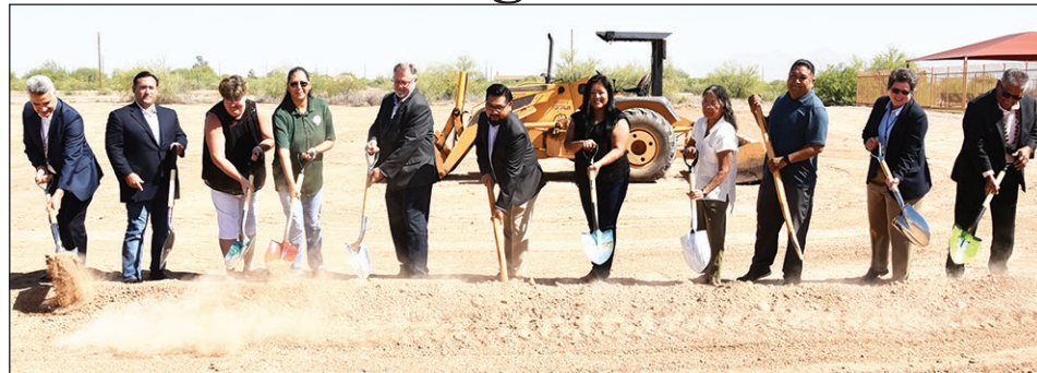
Councilmembers, Community managers, partners and departments break ground with shovels in hand at the PALS housing site on May 9. Some of the shovels used for the groundbreaking were painted by residents and group home staff.
