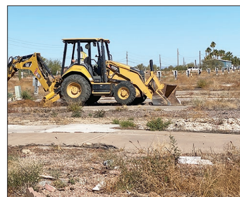
Equipment is used to dig through the site to remove harmful materials.
